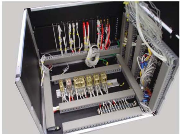
ITA with the Top Cover open and front panel removed to show wiring
