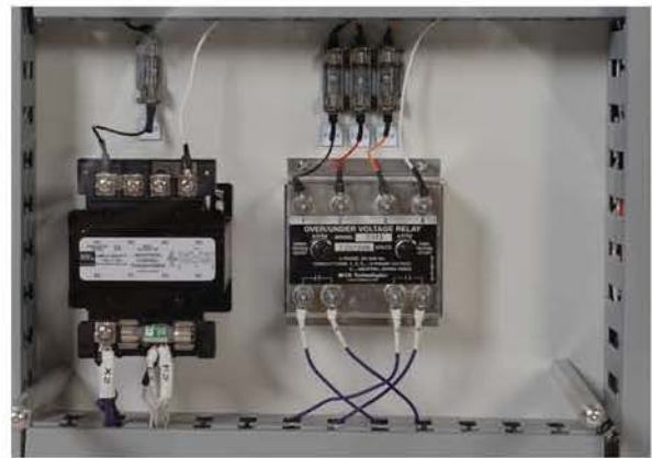
Close-Up of 3 Phase 400Hz AC Input Voltage Monitor to immediately disconnect Input Power to the UUTs if the Input Voltage is out of limits
