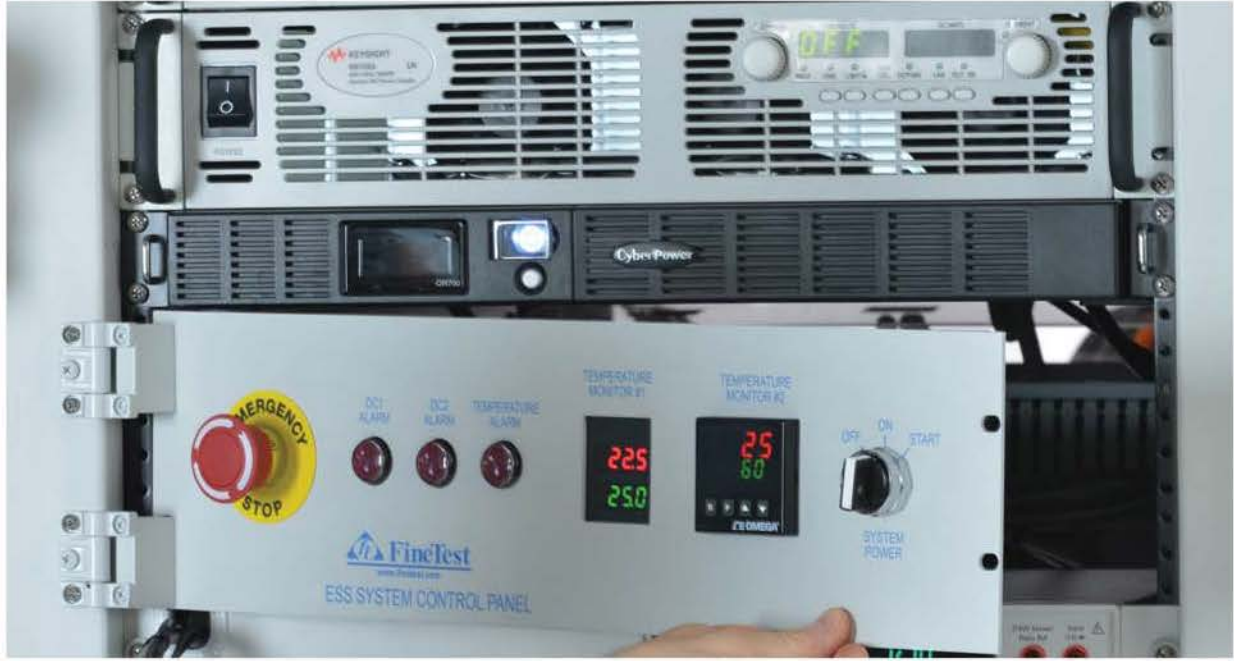
Hinged ESS System Control Panel with Dual DC Input Voltage Monitors and Two Chamber Temperature Alarm Circuits
