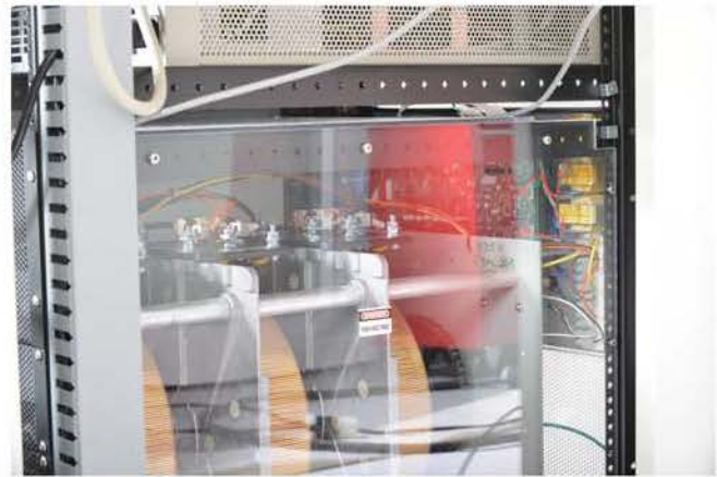
3 Phase 400 Hz Motor Driven Transformer
