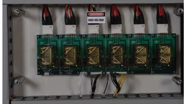
Close-Up of 6 Relays to switch AC Input Voltage On/Off to the UUTs for AC Cycling Tests
