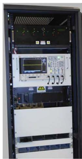
Fixture with added HV Loads and Scope
