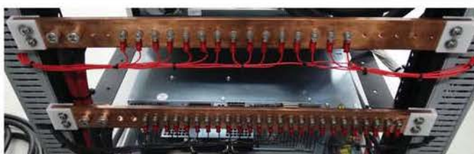
Close-Up of DC Bus Bars
